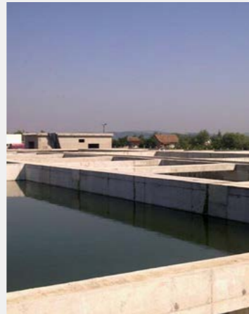
WASTEWATER FACILITY ROMANIA
